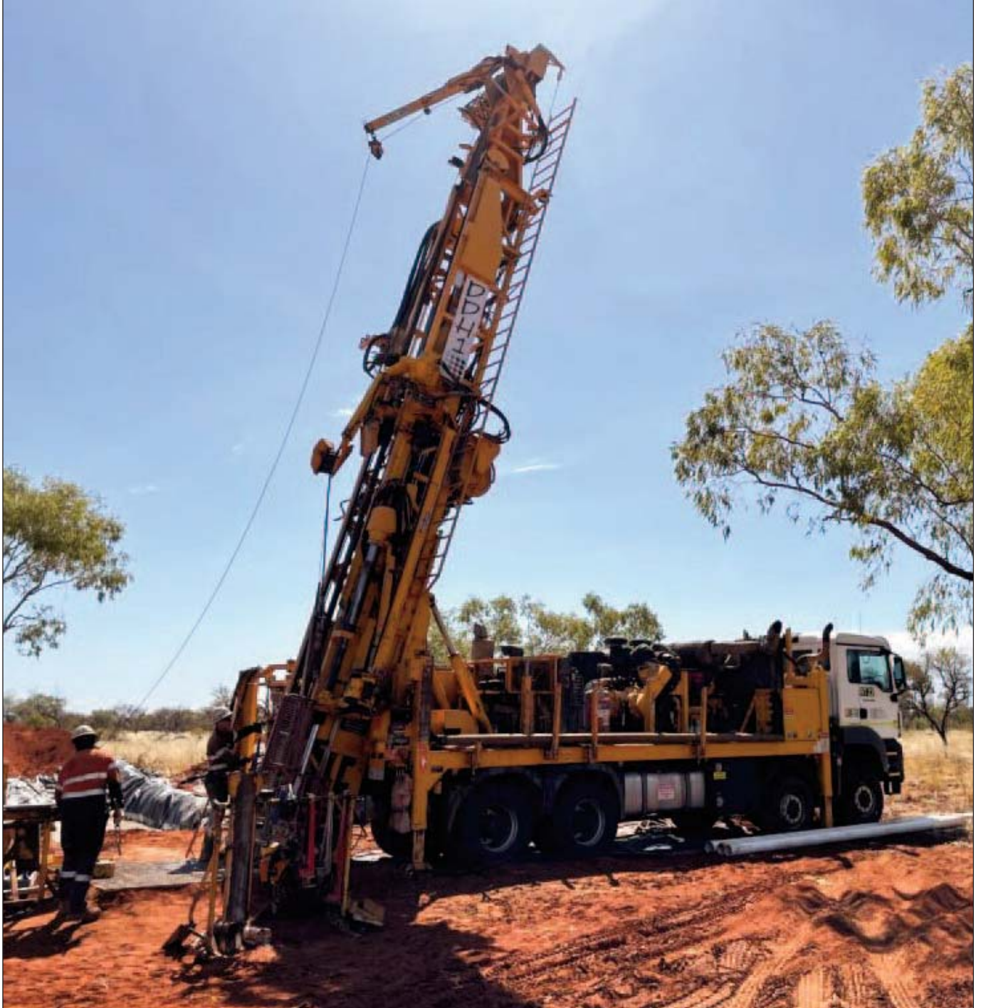
Pictured: A drilling rig at Browns Reef near Lake which has been producing positive results.
